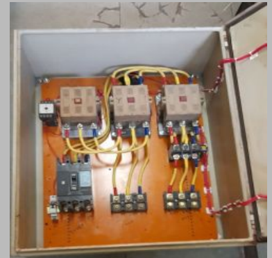
Star Delta Starter Control Panel
