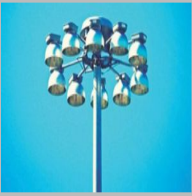
Stadium High Mast Light Pole
