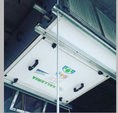
Ceiling Suspended Ahu Unit
