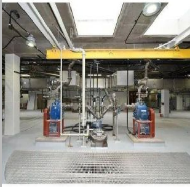
Stp Plant Air Ventilation System
