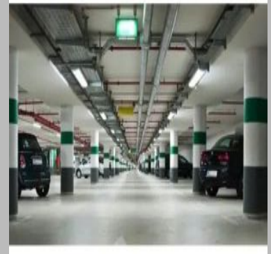
Basement Ventilation System
