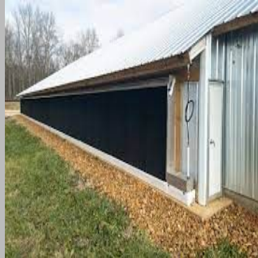
Poultry Cooling System
