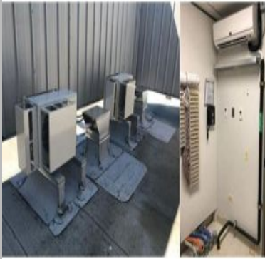
Server Room Cooling System
