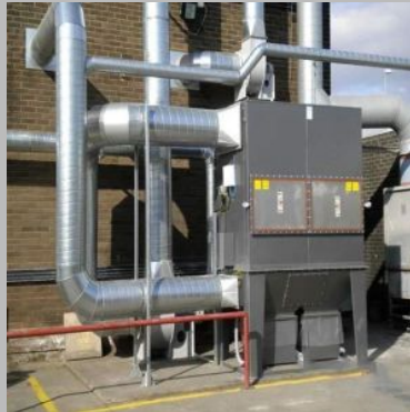
Fume Extraction System
