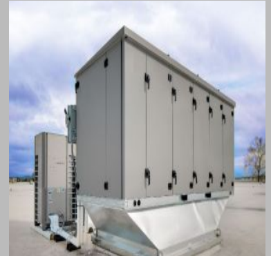
Dedicated Outdoor Air System
