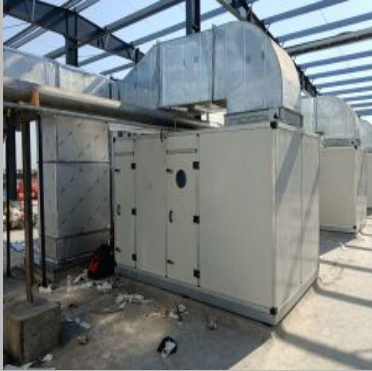
FLOOR MOUNED AHU UNT
