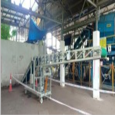
Truck Loading Conveyor
