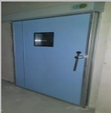
Lead Lined X Ray Room Door
