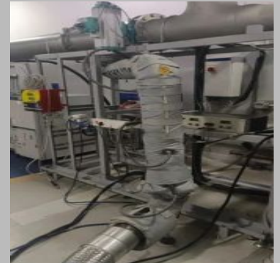
Thermal Insulation Irregular Machine Jacket
