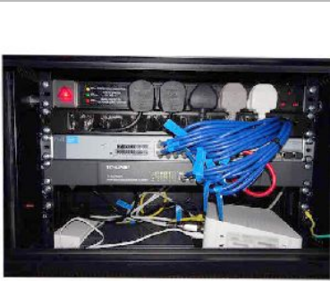
Server Networking Rack
