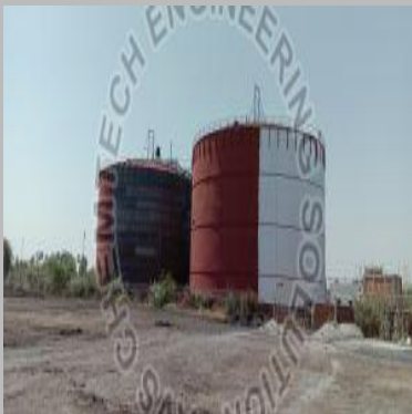
30m X 22m Dia Storage Tank
