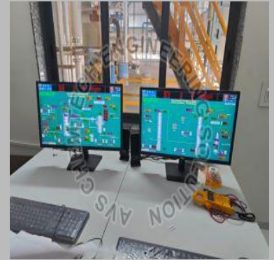
DCS System Formaldehyde Plant
