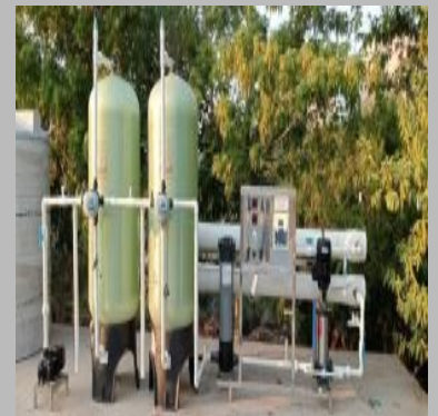
Industries R O Plant
