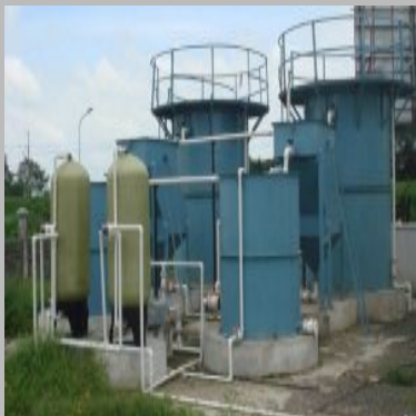
Effluent Treatment Plant
