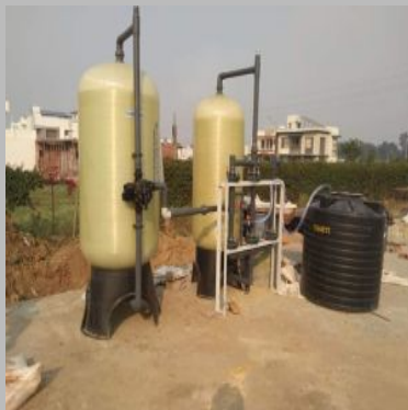
Water Softener Plant
