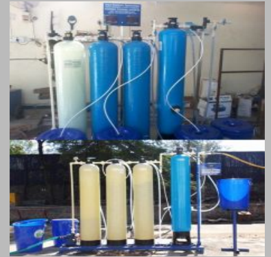
Mix Bed Plant
