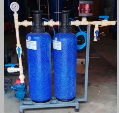
DM Water Plant
