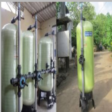
Water Softener Plant
