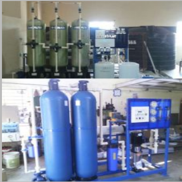
Reverse Osmosis Plant
