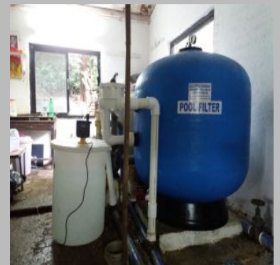
Swimming Pool Filtration Plant
