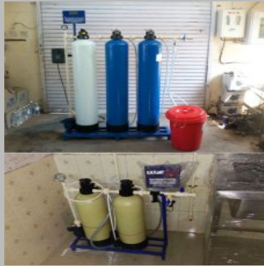
Automatic Demineralization Plant
