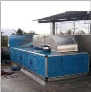
air handling unit
