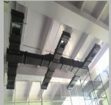
Air Conditioning Duct
