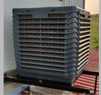
Centralised Air Cooling System
