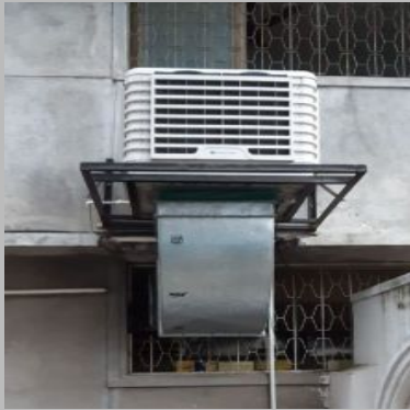
Central Cooling System
