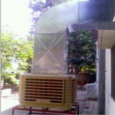
Evaporative Air Cooling System
