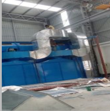
Air Inlet & Exhaust Duct
