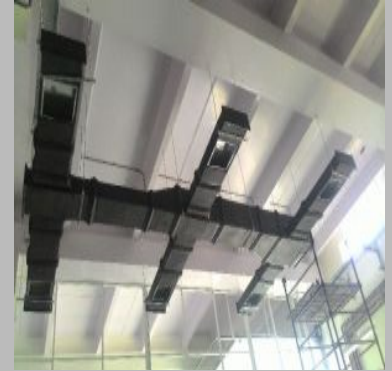
Air Conditioning Duct
