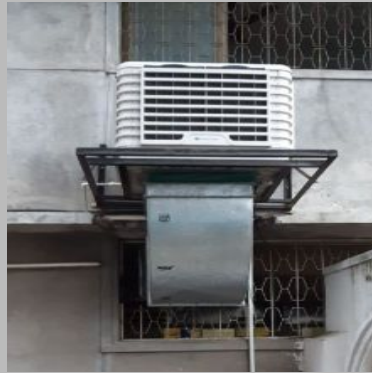
Central Cooling System
