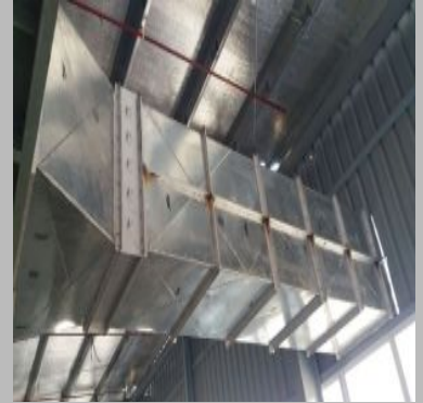
GI Air Duct
